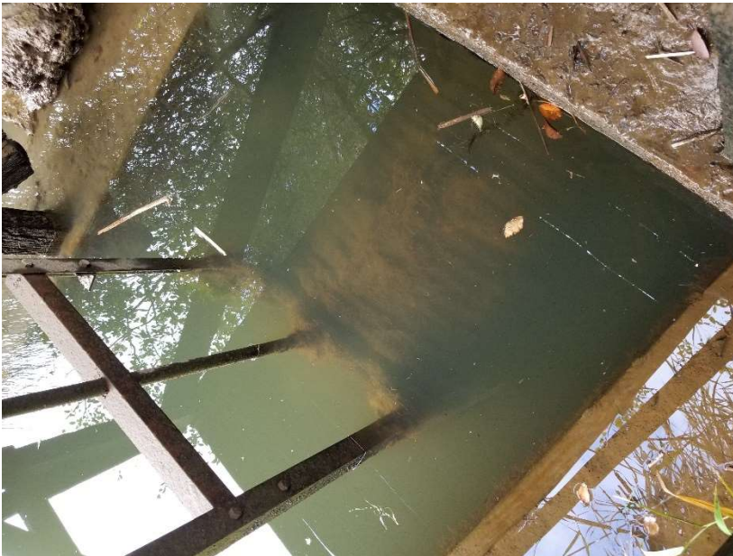
Figure 5. Barn Field water control structures on waterward side of the dike. Culvert with tidegate on end and frame for raising with screw mechanism.
