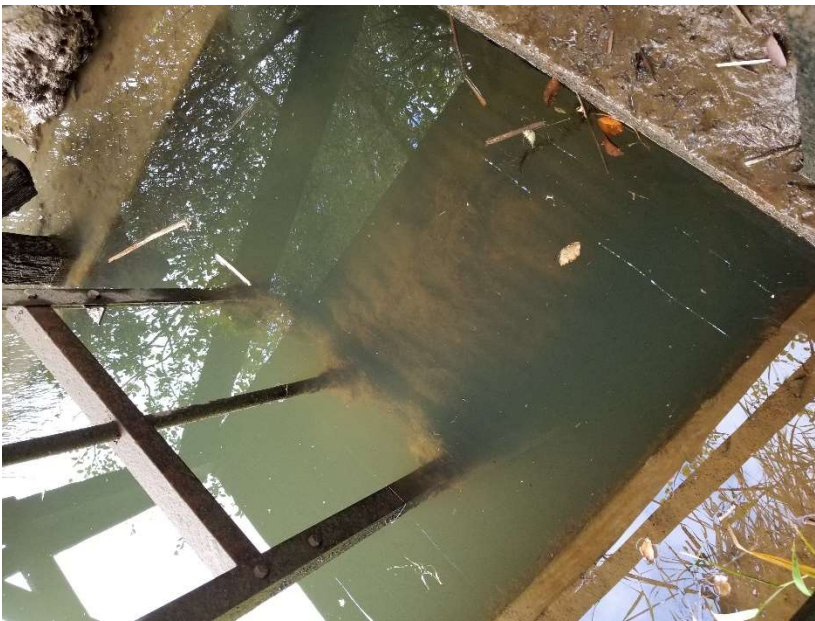
Figure 5. Barn Field water control structures on waterward side of the dike. Culvert with tidegate on end and frame for raising with screw mechanism.
