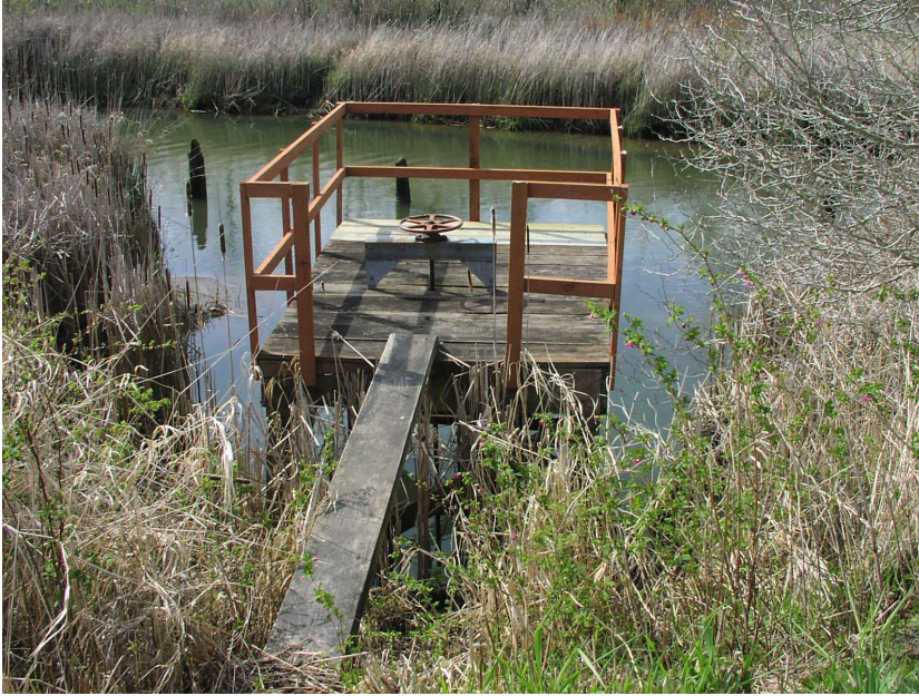
Figure 4. Barn Field water control structures on waterward side of the dike. Footbridge to platform with screw gate controls.
