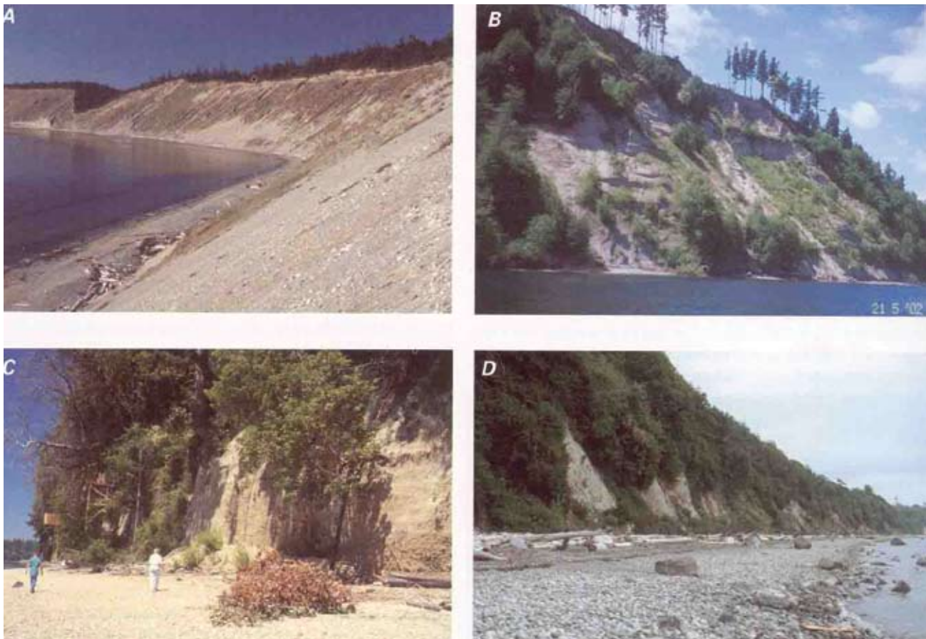
Figure 9. Common bluff configurations in Puget Lowland (from Shipman 2004). A, high bluffs composed of poorly consolidated outwash gravels. B, 300-ft high bluff in Tacoma consisting primarily of advance glacial outwash. C, ~45-ft bluff in southern Puget Sound composed of compact sediments that form near vertical slope, also note colluvium at toe of bluff. D, Northern Puget Sound bluffs, exhibiting steeper bluff toe profile, with toe erosion.
