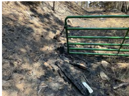
Figures 3, 4, 5 & 6: (Top left.) In some locations, wood posts used to mount access gates disintegrated leaving behind empty holes with nothing to keep the gates in place. (Top right.) In other locations, gate posts remain standing, however, severely damaged posts no longer securely hold mounting hardware. (Lower left.) With the wooden gate posts completely burned, staff find other ways to temporarily keep gates upright. (Lower right.) Compromised gate functionality make propped gates a safety hazard, however, still used to help detour the public from access to closed burned areas. Gate replacement is a priority. . Photo credits, Bob Dice, Chief Joseph Wildlife Area Manager
