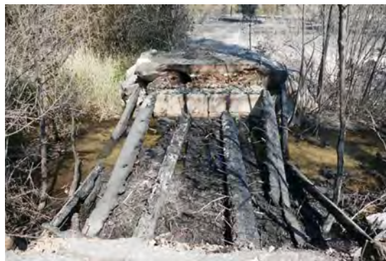
684 Eastside Chewuch Rd. Winthrop, WA 98862 - Dammann Dairy historic site – The bridge used to cross the irrigation canal was badly damaged in the Cub Creek 2 fire. This small bridge is crucial to the local ditch company as it's their only way across the canal and its loss will impact upcoming maintenance projects. (Photo courtesy of Methow Wildlife Area Manager, Brandon Troyer.)
